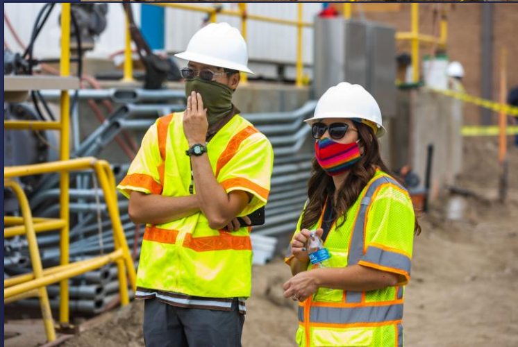
Greg Avenue Pump Station, Expanding Flexibility of Distribution System
